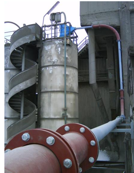
Pneumatic conveying circuit with anti-abrasion bends and end receiver at arrival.
