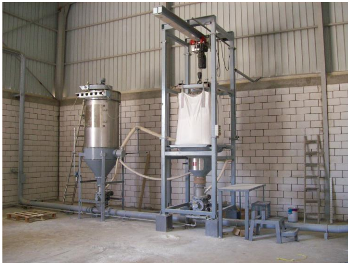
Pneumatic conveying system including a Big Bags emptying station and a Fines collecting filter and their reintroduction into the circuit (clean station)
