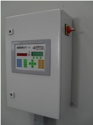
Control command cubicle IP55
